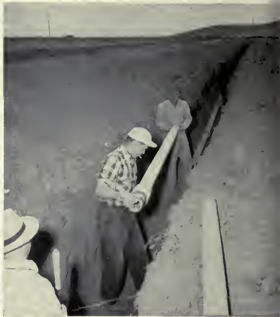
THEY DID THE WORK.—Settler Art Johnson, foreground, holding pipe, W. C. McDonnell, center, and Clarence Schwabke working on ditch in background, helping to bring their own domestic water to the Westmont Acres Water Association's part-time units near Soap Lake, Wash., on the Columbia Basin project.
